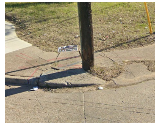
Ramps not ADA compliant
