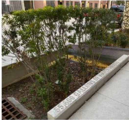
CG-1.0 Built example of bioretention planter in Houston
